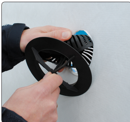
Squeeze the grill of the KimaAir inside/out and push through the hole so that the underlay will be between the grill (out) and underpart (in) mount the underpart, whilst holding onto the strip.
